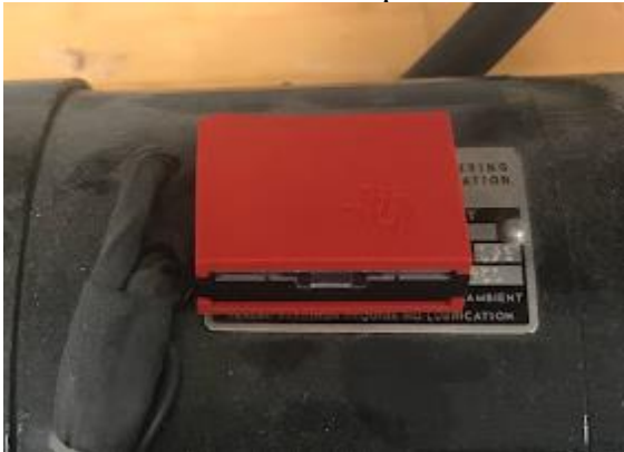
Sensor-Tag location over motor 1
