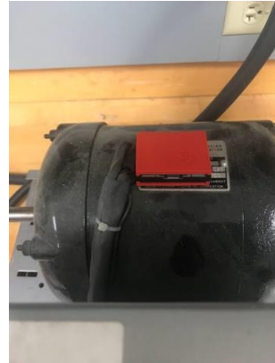
Sensor-Tag location over motor 1
