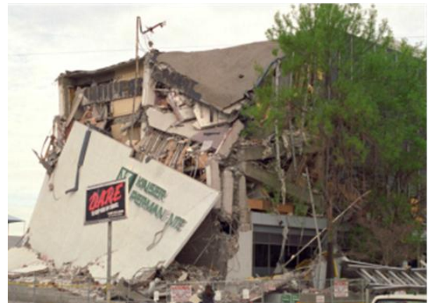
Figure 1. Structure collapse because of failure of deficient beam-column joints, Kaiser Permanente Building, Northridge earthquake, 1994.
