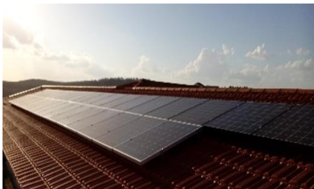
Figure 3: University of Évora's PV installation.
