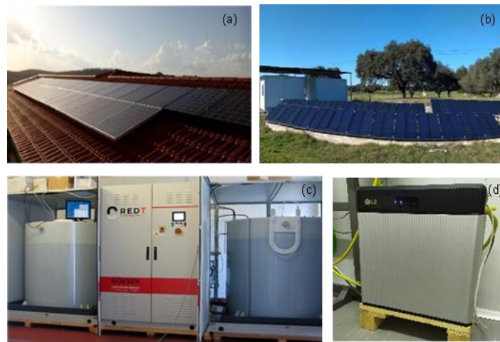
Figure 1: (a) Solar photovoltaic installation 6.7 kWp; (b) Solar photovoltaic installation 3.2 kWp; (c) VRFB redT 60 kWh; (d) LIB LG Chem Resu 10, 9.8 kWh.
