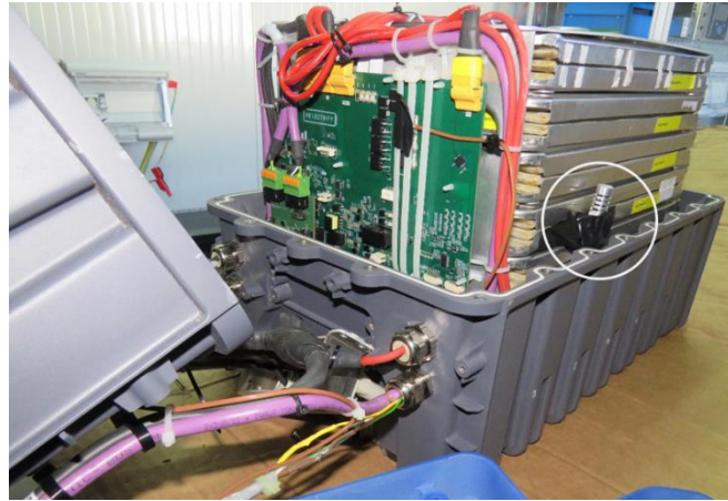
Figure 18. A humidity sensor was installed next to the battery cells and inside the housing of one of the second-life lithium-ion batteries (marked with a white circle to facilitate reading).
