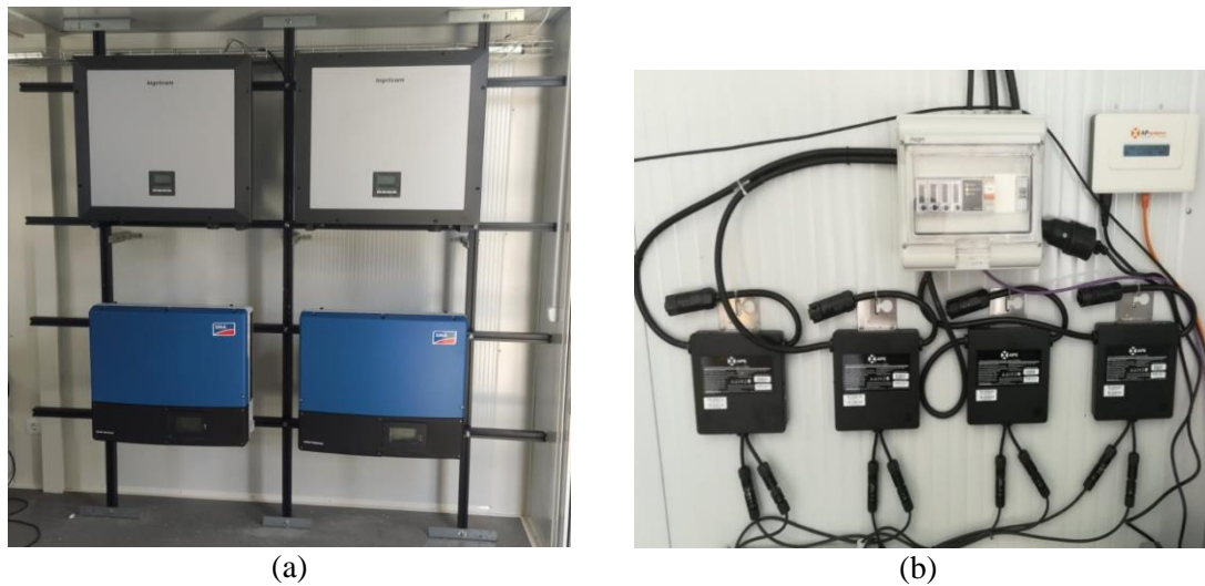
Figure 22. (a) Inverters of the solar PV trackers. The two above inverters are SMA Sunny Tripower (STP) 20000TL-30 and STP 25000TL-30 [35] inverters, and the two below are Ingeteam Sun 3play 20TL inverters [34]. (b) Repaired modules' microinverters from APsystems YC250-EU [36].
