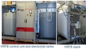
VRFB control unit and electrolyte tanks
