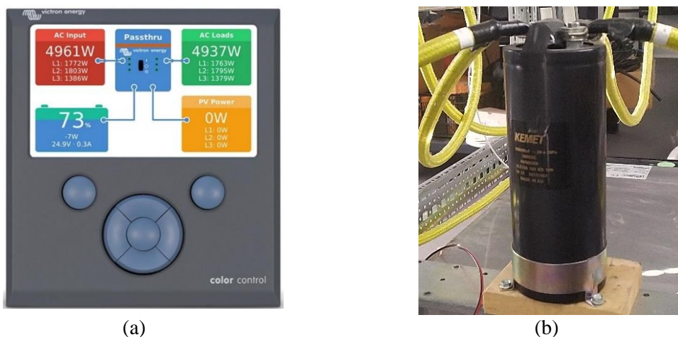
Figure 15. (a) Victron Color Control GX [12] as the communication interface with the Victron Multigrad inverter/charger; and (b) Capacitor installed to stabilise voltage to the battery pack.
