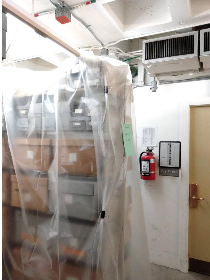
Collections in the stacks covered with plastic, in preparation for new heater installation in the ductwork.
