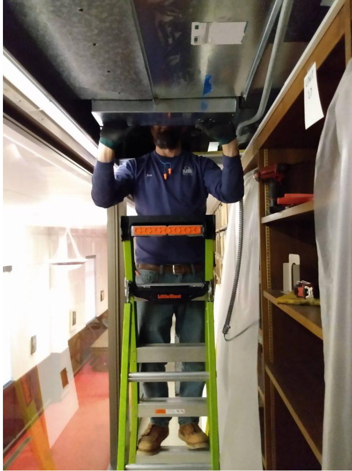
Contractor installing a new heating unit in the ambulatory area of the second floor North Gallery stacks.
