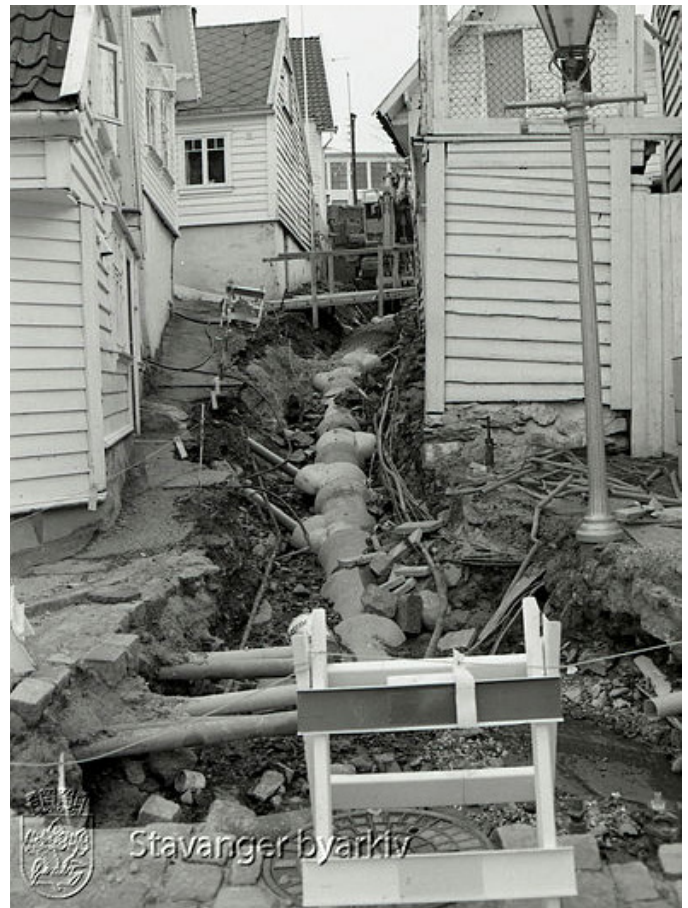
Fig. 64. The construction of sewage pipe down Andasmauet in 1987 (Foto: U.B. Stavanger Byarkiv)
