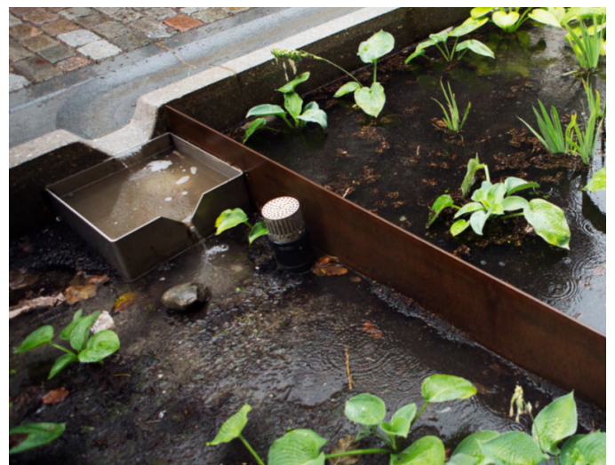
Fig. 24. The gardens are sitting in the ground, water goes through a sedimentation chamber to reduce sediments in the bed (Egeberg et al., 2021, p. 21).
