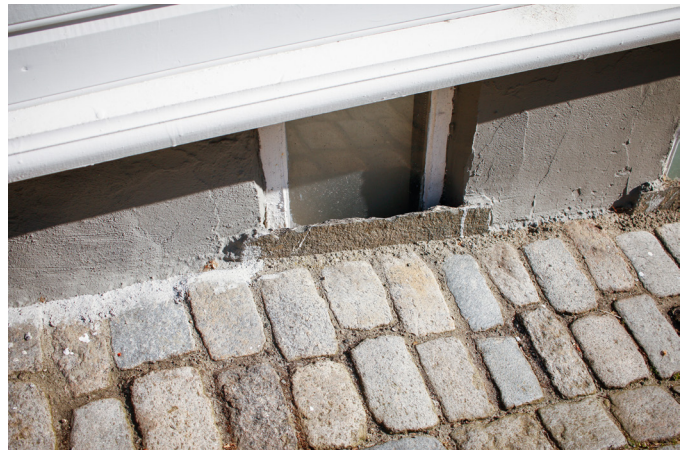
Fig. 92. A small intervention can be enough to keep the water out of cellar (IP, 2023)
