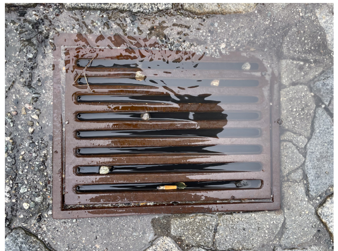
Fig. 3. Clogged storm drains in the upper parts of Gamle Stavanger (IP, 2023).
