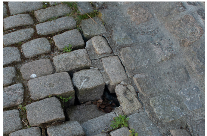
Fig. 44. From left to right the transition between permeable cobblestone with dirt and sand filling to impermeable cobblestone using a cement mix. Trying to protect the foundation of a heritage building from water damage in Straen. The supporting mass of the cobblestone is however scrubbed away from eroding water under the stones and the pavement is falling apart, feeding water under the protective measure (IP, 2023)
