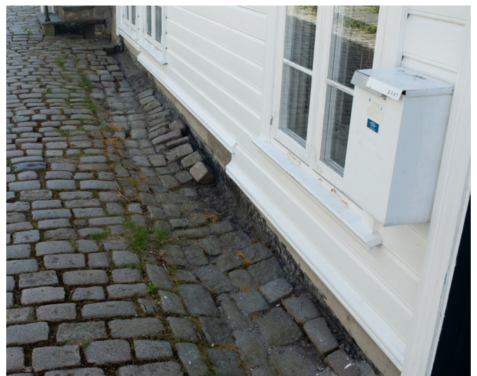
Fig. 86. The edge here has been washed out, by rain events or other kinds of erosion (IP,2023).
