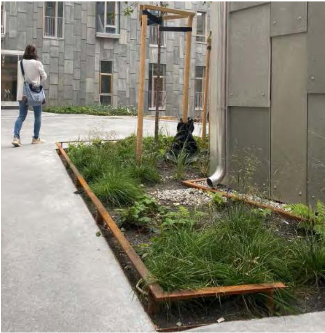
Fig. 19. A rainbed situated close to a building, a membrane is protecting the underground structures from water damage. water can flow directly into the bed from all sides because it does not have a raised edge (Egeberg et al., 2021, p. 35).
