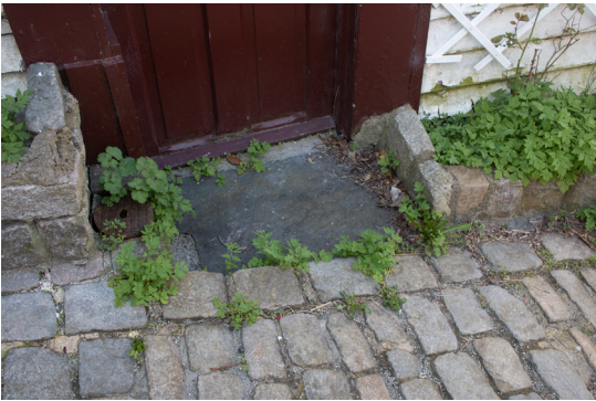
Fig. 89. An entrance in Andasmauet, that may be exposed to water problems (IP, 2023).
