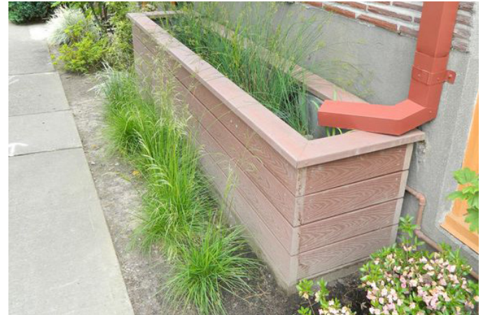
Fig. 10. A raised rainbed can provide great potential for water retention and infiltration (New Jersey Future, n.d.).
