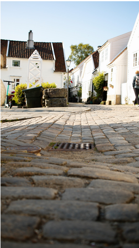
Fig. 87. This little bump interferes the water changing the direction of water into the drain (IP, 2023).
