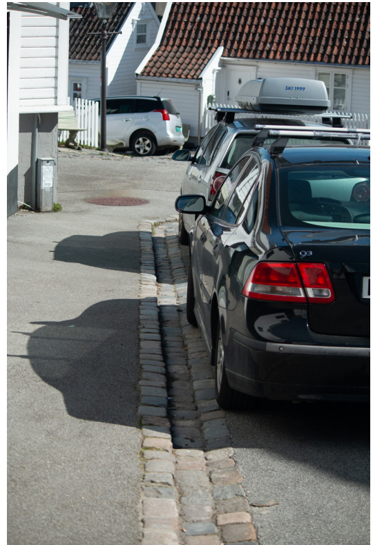
Fig. 88. On the side of the road there is a little cobblestone edge sitting a little lower than the rest, the stone will slow down the water, and lead it along the curb (IP, 2023).
