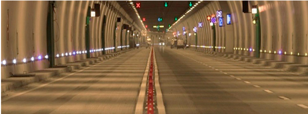
Figure 4.1: An Example of Flickering of Lights in Road Tunnels by (Peña-García, 2018)
