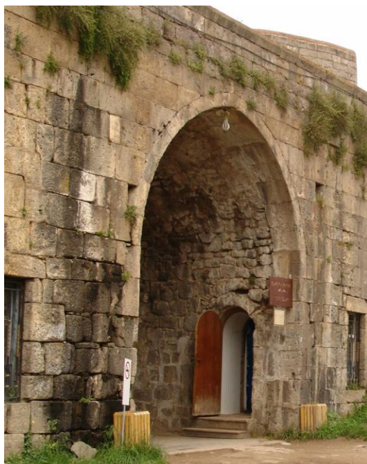
Fig. 8. The vaulted roofs of the auxiliary rooms adjoining the fortified walls in Tatev Monastery, Source: own studies.
