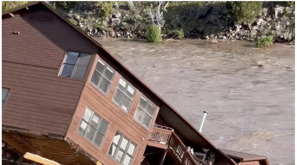
Photo Credit: “Yellowstone River Swallows Housing for National Park Employees.” K2 Radio. June 13, 2022.
