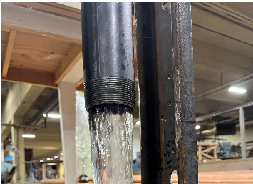
Figure 3 – 2-inch diameter, steel pipe nipple.
