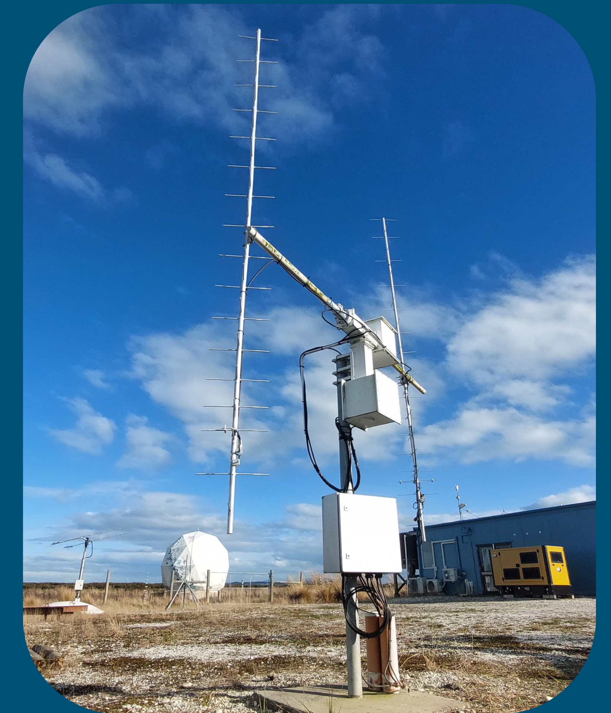
Receive station Awarua Satellite Ground Station, New Zealand
