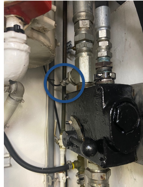
FIGURE 3: HYDRAULIC SENSOR (CIRCLED) INSTALLED ON GROUND FISH VESSEL. PHOTO CREDIT: CHLOE SWICK
