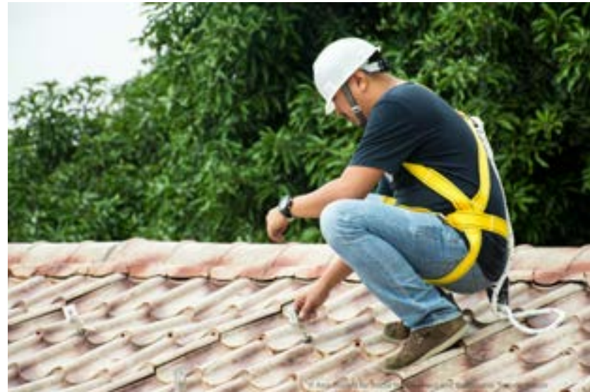
Clifford was one amongst the 2 million unemployed Filipinos in 2018. The Rooftop Solar PV System Installers Training Program, under the project AccessRE, provided Clifford with new avenues for learning, on-site installation training, and access to employment opportunities in the solar industry. (Photo: ASSIST)
