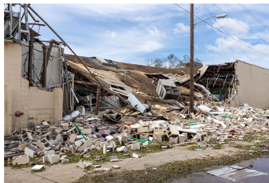
LAKE CHARLES, LA - AUGUST 27, 2020: Hurricane Laura makes landfall as a category 4 storm causing severe hurricane damage to buildings in downtown Lake Charles.
