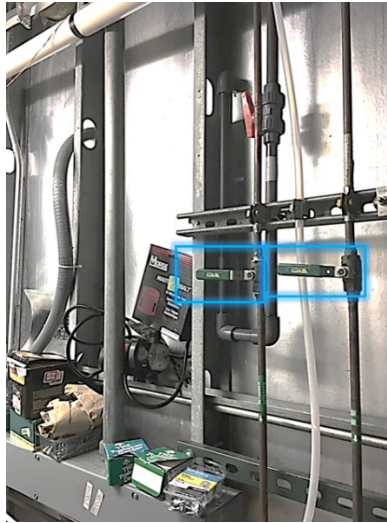
Figure 142. Valves to be opened in the chase bay behind the chemcut.
