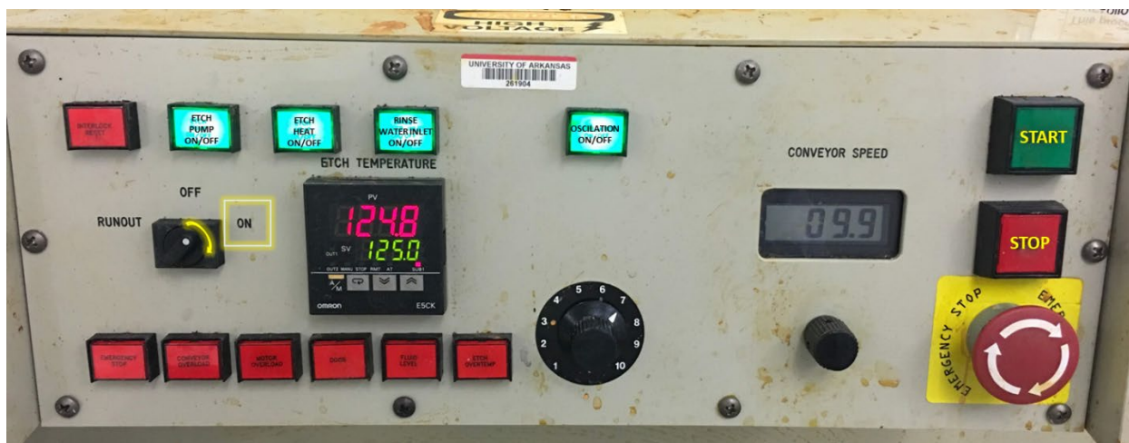
Figure 132. Chemcut spray etcher control panel
