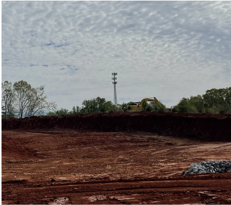
Figure 3.19: Cellular Tower at Central Site
