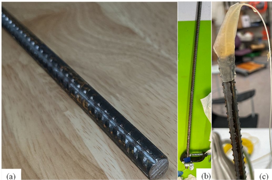
Figure 3.19. Procedure for installing FBG fiber in rebar (a) 1.5x 1.5mm slit on rebar, (b) laying and clamping of fiber on rebar, and (c) conical urethane cast on the splice for protection
