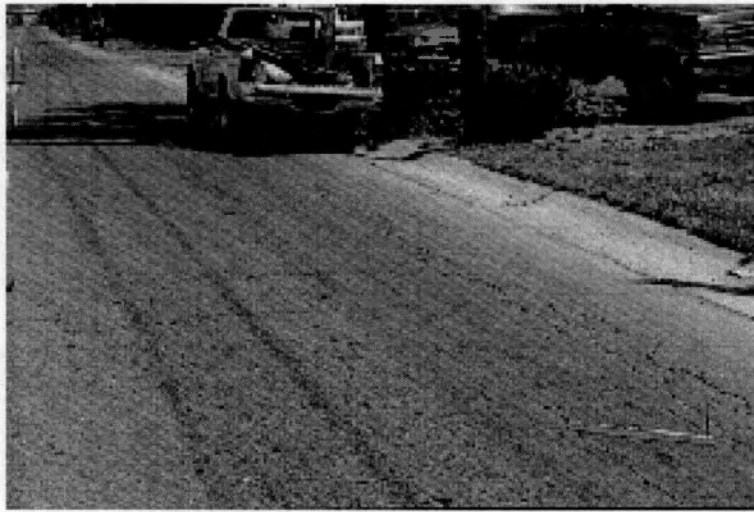
Figure B.2: Moderate severity Fatigue cracking.
