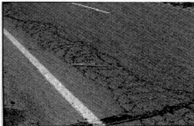
Figure B.3: High severity Fatigue cracking.
