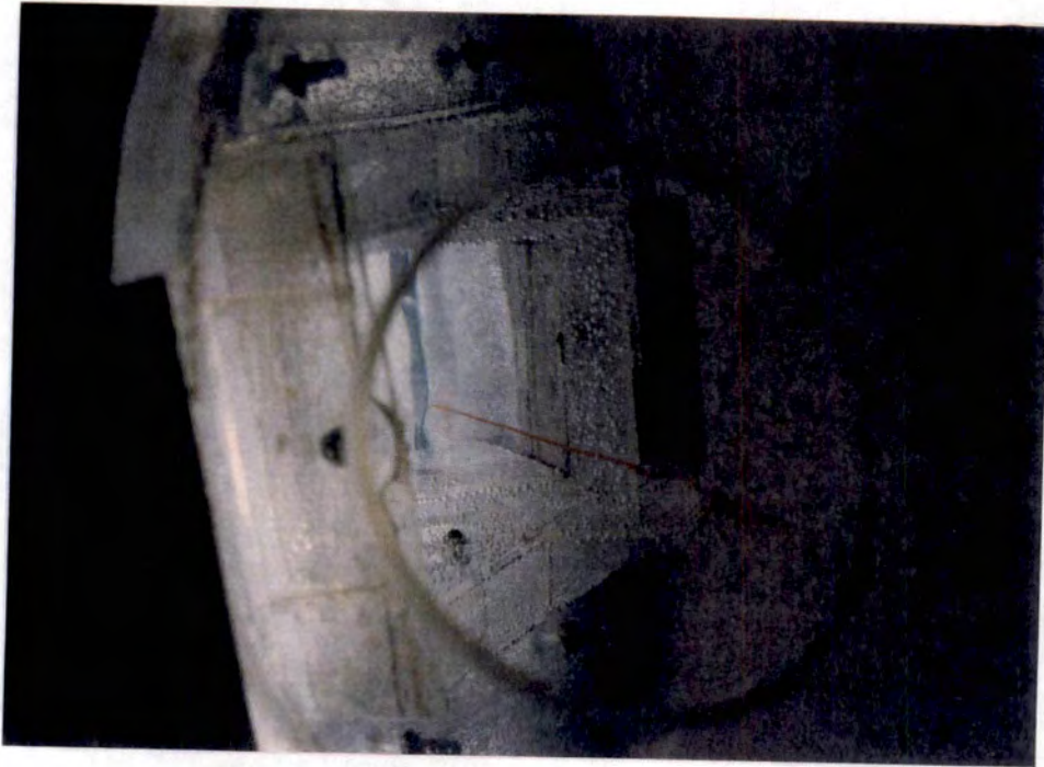
Zone 1, View Upstream into Nozzle Exit
