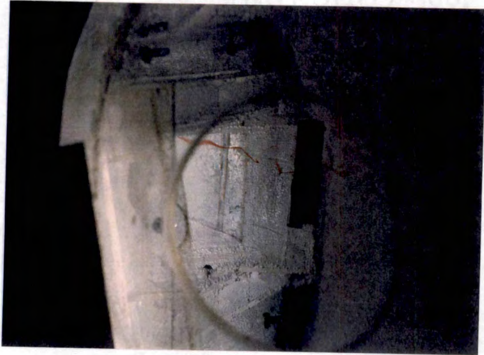
Zone 3, View Upstream into Nozzle Exit
