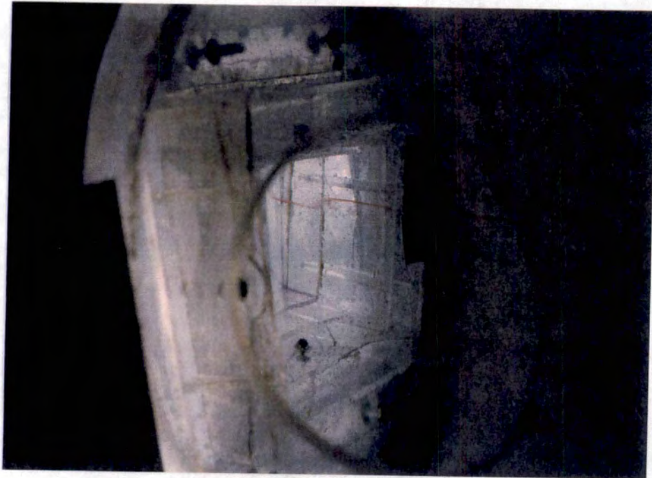
Zone 3, View Upstream into Nozzle Exit
