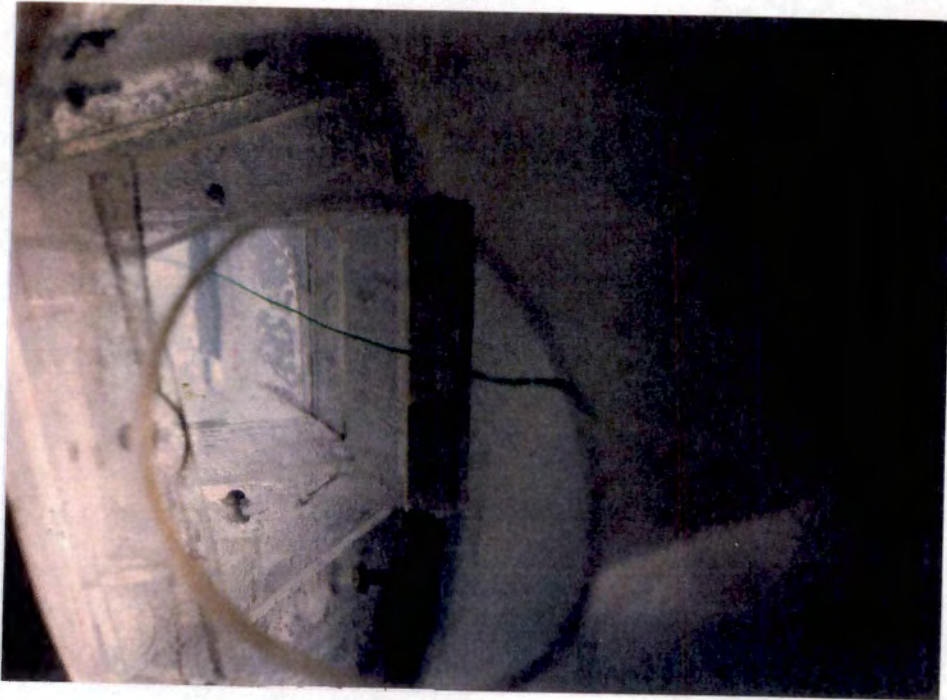
Zone 2, View Upstream into Nozzle Exit
