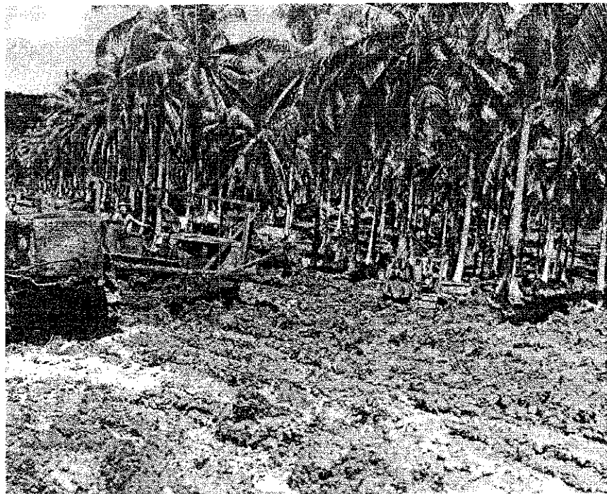
The nature of the terrain and the difficulties of construction in the Russells are evident in this photo of road construction. Official USMC photo.
