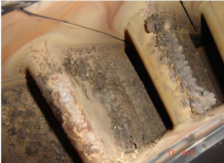
Figure 1.4-1 Deposition of first stage vanes of utility gas turbine after approximately 8000 hours of service. Firing temperature 1150°C. Source: [36].
