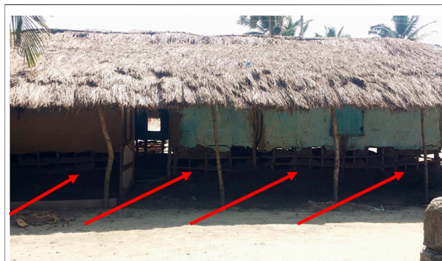
FIGURE 3 | A house in Woarabeba destroyed by the recent flooding even in November 2019 (Arrows pointing to base of the building damaged by flood waters).
