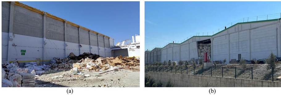
Fig. 30 Damage of precast buildings in Turkoglu OIZ a precast tapered beam failure owing to the loss of support, b cladding panels due to panel-to-structure failure
