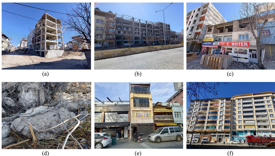
Fig. 16 a and b Two buildings with different construction practices, c a building with an added third story, d poor concrete and plain reinforcement, e and f no separation between buildings
