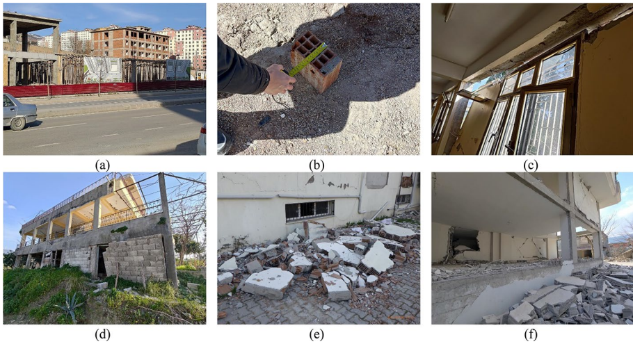
Fig. 20 a Two buildings of one construction project, b a typical brick, c and d brick walls popped out of frames, e brick walls fallen down, f beams and columns were almost intact but brick walls seriously cracked
