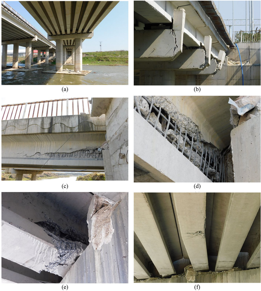
Fig. 28 Bridge 2. a overall view from underneath the bridge, b failed exterior shear keys, c damage at girder ends, d concrete damage and spalling at girder ends, e damaged and twisted girder end, f bent girder
