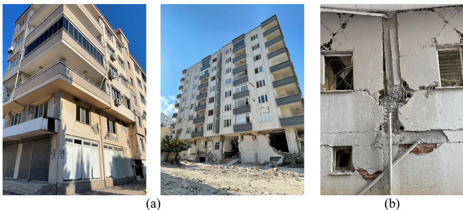
Fig. 22 Residential building damages a due to overhangs, b captive/short column due to strong infill walls
