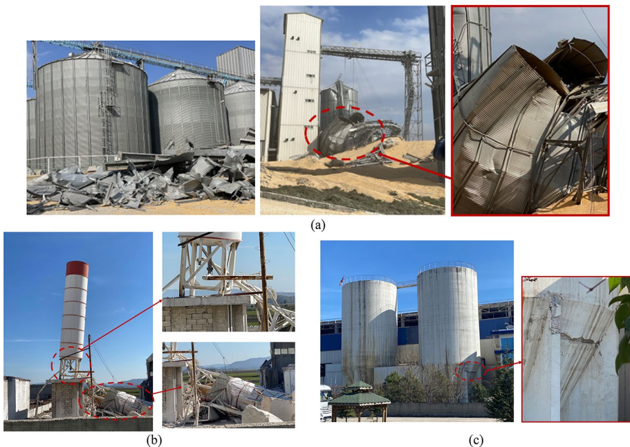
Fig. 34 Damage of silos a corn silos, b total collapse of a slender metal silo due to brittle welded connection, c concrete spalling on silos
