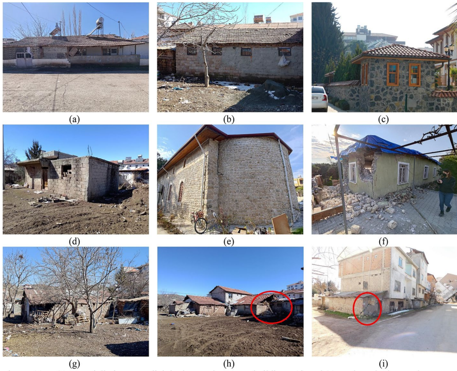
Fig. 23 a–c Essentially intact or slightly damaged masonry buildings, d and e moderately damaged masonry buildings, f–h severely damaged masonry buildings, i a pure sliding mode of failure mechanism of a brick wall
