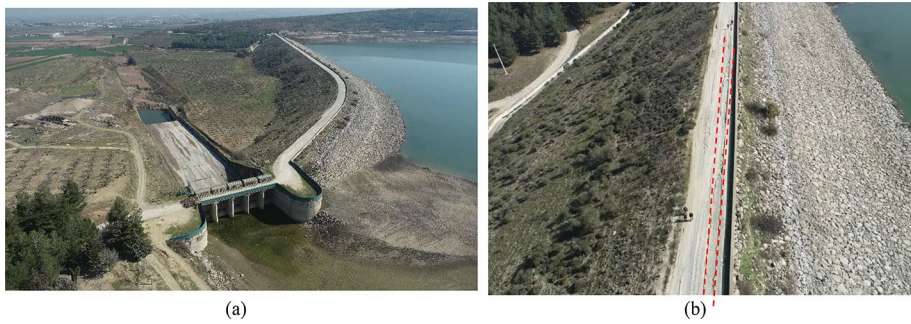
Fig. 11 Aerial pictures of the Yarseli dam (36.194290N, 36.329264E): a Overview; b Cracks in the crest
