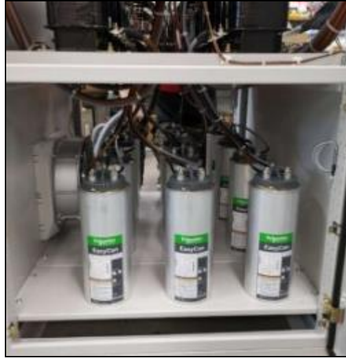
Figure 5.22: Image of capacitor bank install (AWE, 2021)
