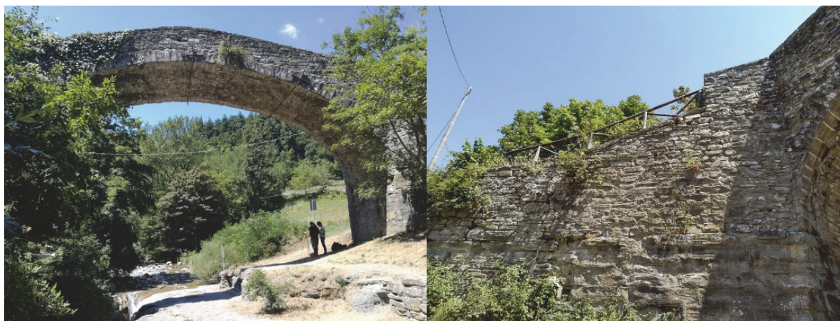
Figure 1: An example of infrastructure deterioration.
