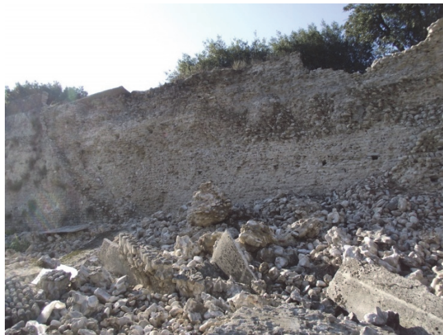
Figure 5: Collapsed portion of the wall, Pistoia
