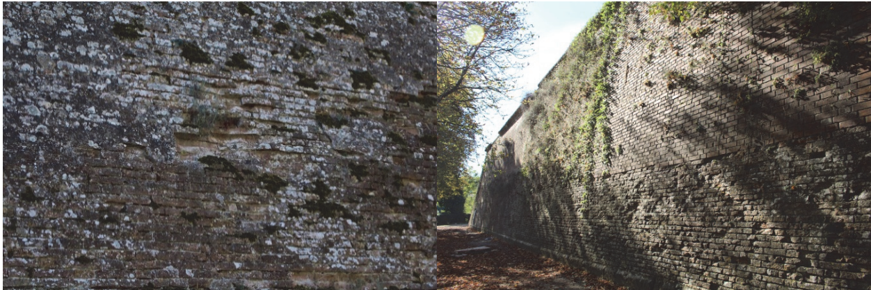
Figure 2: Examples of degradation due to moisture
