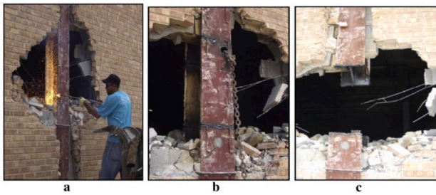
Fig. 10. Dynamic column removal in existing steel frame building; (a) torching of the removed column, (b) column ready to be pulled out, and (c) removal of the column, as reported in [56].
