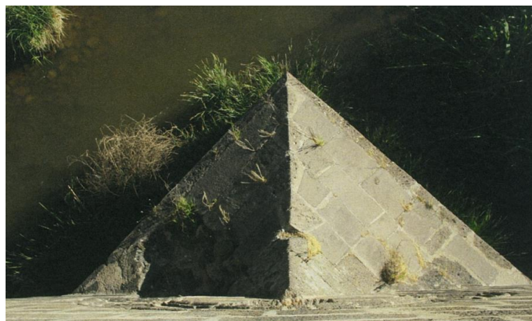
Figure 13. Breakwaters suffer from vegetation and deformation
