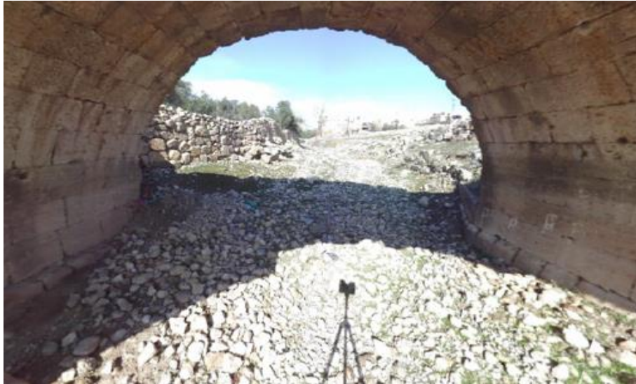
Figure 6. Erosion on the foundations of Bridge
