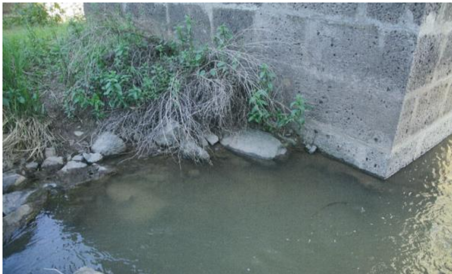
Figure 7. Large stones and trees are carried onto the bridge
