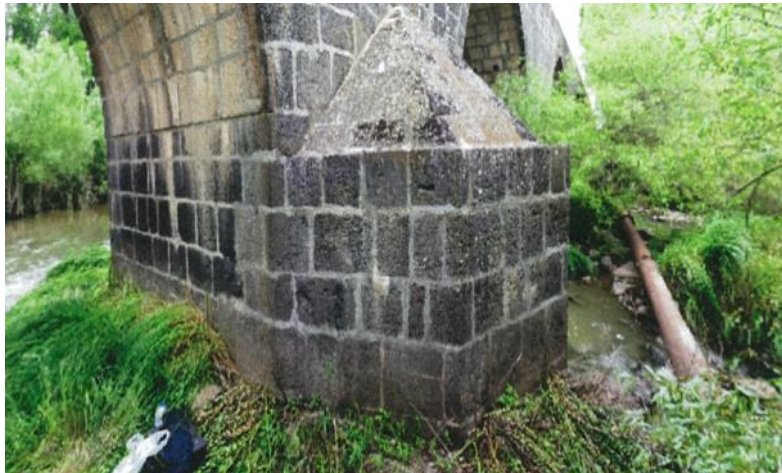
Figure 9. Growth of vegetation on the piers
