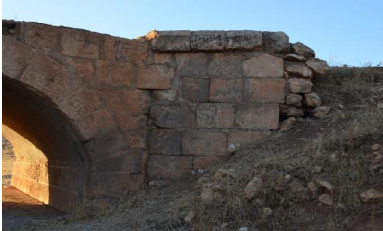
Figure 8. Damaged abutment of bridge
