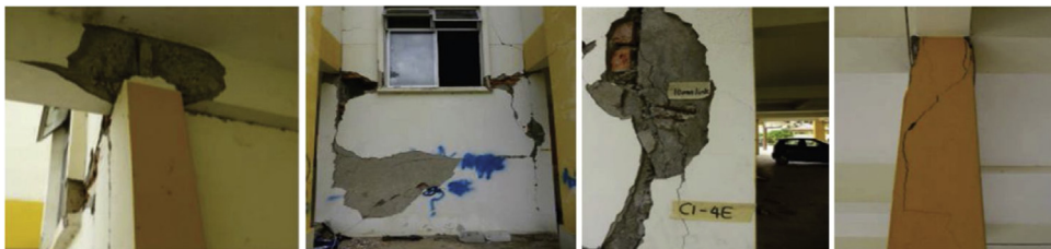
Fig. 7. Field damage observation after Ranau seismic event [32].
