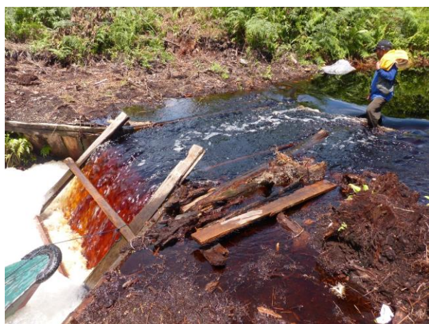
Box dam on upper Sungai Buring, near Buring patrol post in the north-western part of SMPP. Constructed in late 2017, photo by W. Giesen on 26 April 2018, by which time the dam had been overtopped and damaged. More details on box dam construction are provided by Dohong et al. (2018).
