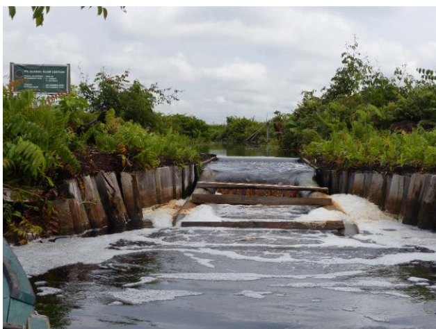
KBG26 on Sei Tembesu Daro in the mid-southern part of SMPP; UTM: X408522/Y9776023. Constructed Sep 2017, photo Apr 2018 by W. Giesen for SMPP. As with most box dams the outer construction is of timber and the centre filled with bags of soil/peat, with a spillway in the middle to facilitate boat access upstream.
