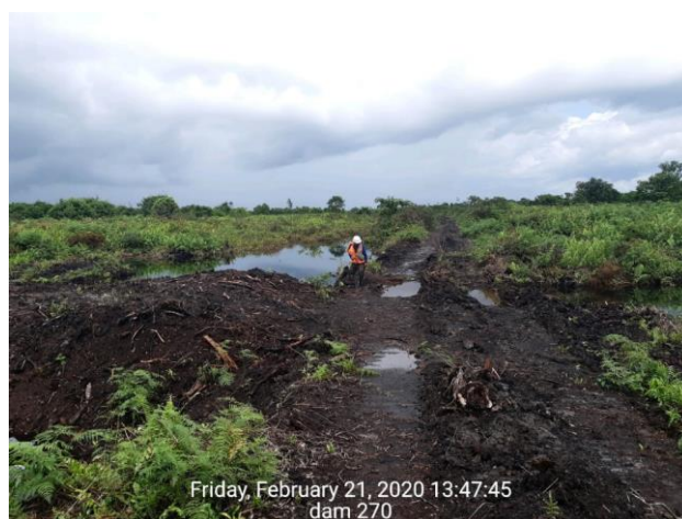
Dam 270, also near Sialang patrol post; UTM: X396303/Y9774668. Constructed Feb 2020, photo 21 Feb 2020 by P. Richardson for SMPP. The canal is almost 3 m wide. More details on compacted peat dam construction are provided by Dohong et al. (2018).
