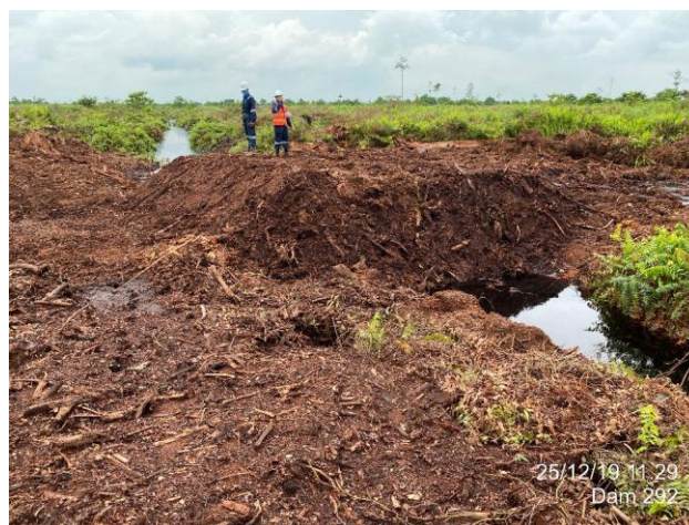
Dam 292, cluster 7 near Sialang patrol post, western end of SMPP; UTM: X397034/Y9775702. Constructed Dec 2019, photo 25 Dec 2019 by W. Boissevain for SMPP. The canal is 2.2m wide but the compacted peat dam (constructed using an excavator) is several times this width and is raised to 128 cm (range 105–170 cm) above the field level.
