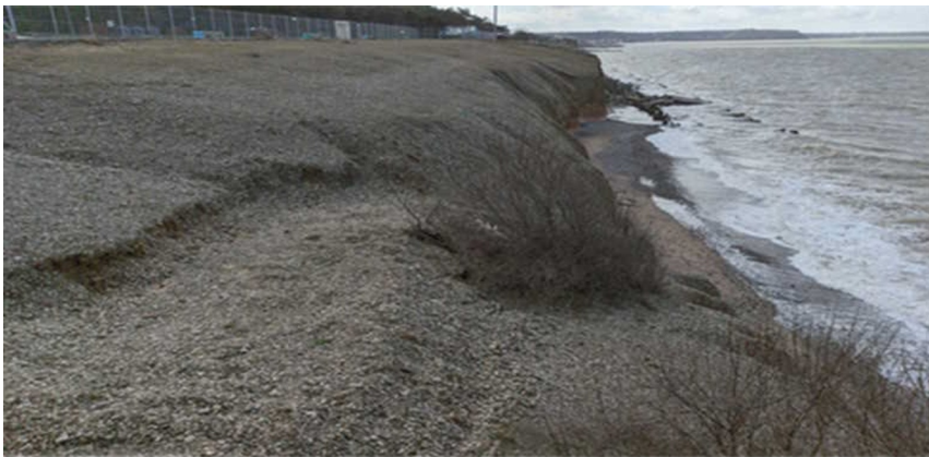
Fig. 8. Destroyed coast protection in the area of the boarding houses "Iskra" of LLC "Ukrtelekom", the pioneer camp "Stroyindustria", shore protection structures of the public beach, boarding house "Minmontazhspetsstroy", boarding house "Volna".
