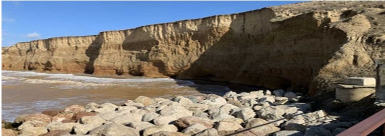
Fig. 1. Abrasive-landslide bank to the north of the reconstruction site.
