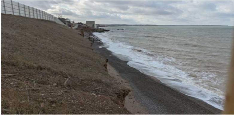
Fig. 3. Natural cliff on the site of destroyed shore protection structures in the area of the boarding house "Rainbow".
