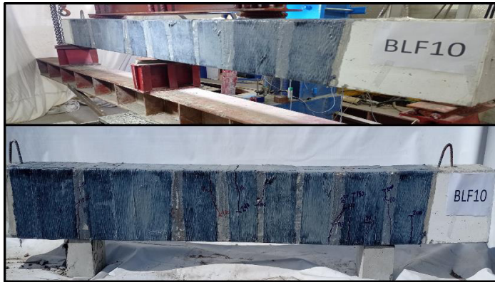
(c) Crack patterns in the tested extended continuous beams at the failure stage (BLF10).
