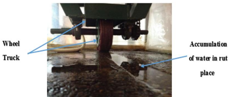
Figure 12: Resulting rutting on the pavement.
