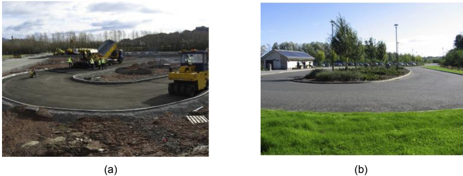
Figure 5: a: Construction of the bus turning circle, b: Bus turning circle 3 years after construction [71].
