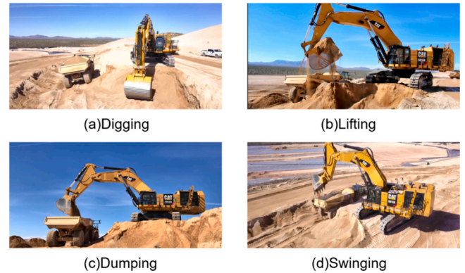
Fig. 2. The four investigated working stages/activities involved an excavator. The involvement of dumper is not essential.
