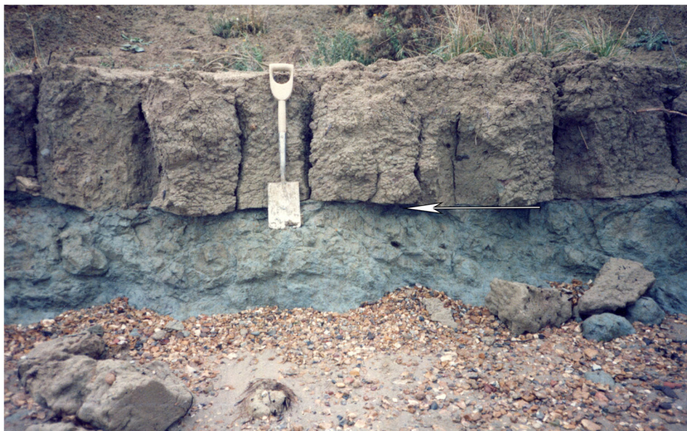
Fig. 2 Lowermost portion of section at Bouldnor Cliff (Isle of Wight, England, UK) from which Eomys teeth were collected. The arrow indicates the position of the ‘ Eomys bed’. Photograph placed at our disposal by R.L.E. Ford (1985)
