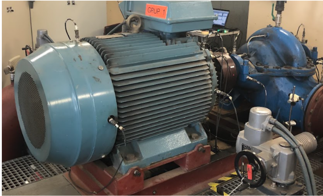
Figure 4.2.1. SG pump with accelerometers installed in the three directions
