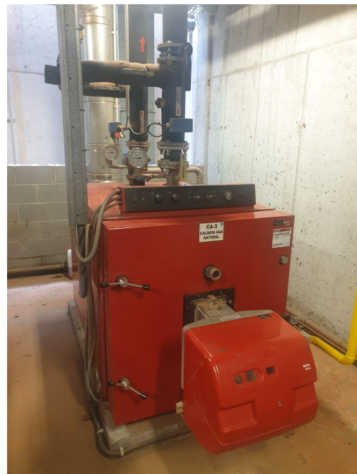
Figure 46. Natural Gas boiler 2
