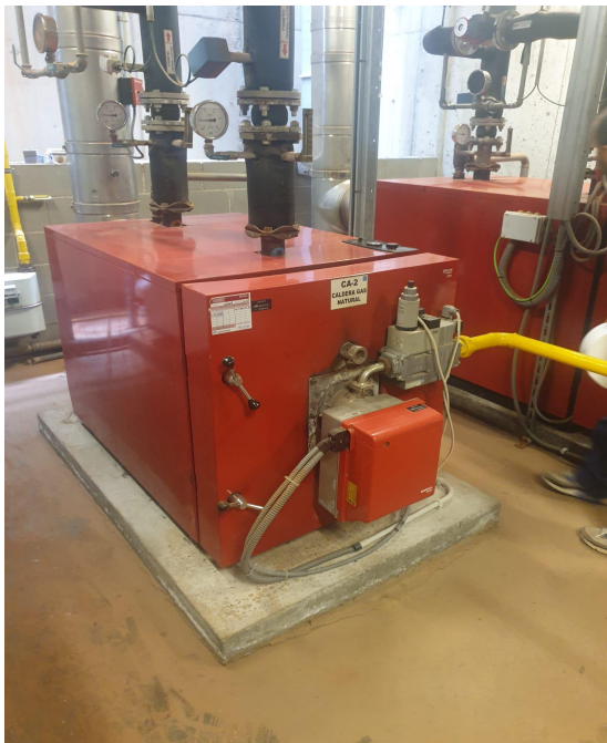
Figure 45. Natural Gas boiler 1
