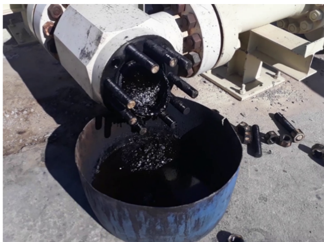
Figure 1. Solid deposits accumulated behind the surface choke.
