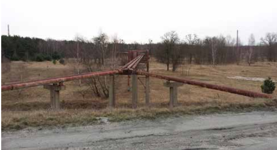
Figure 1. The pipeline drained a mixture of ash and slug to the landfill in EDF Toruń SA
