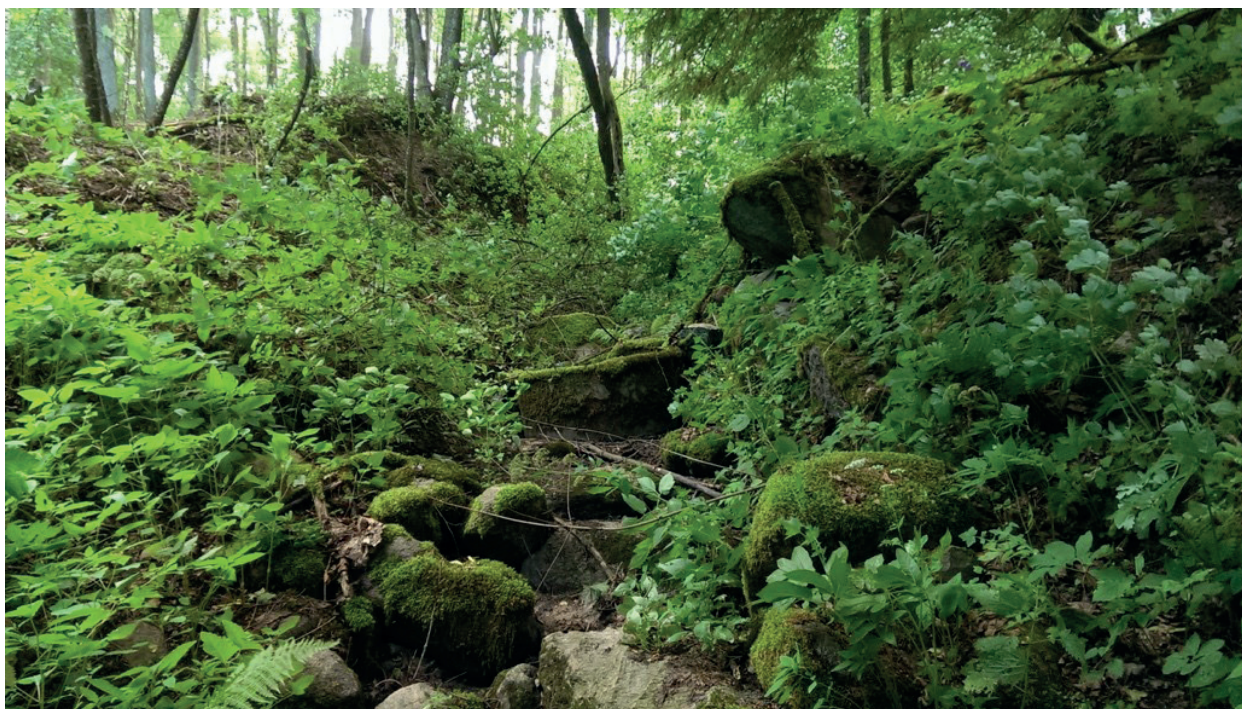
Photo 1. Destroyed culvert on dirt road between Lake Niskie and Lake Wysokie. Foreground: scattered concrete culvert rings (July 2019).
