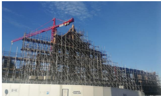
Figure 84. Part of the old Victorian Belmont Works factory building covered by scaffolding, 2019.
