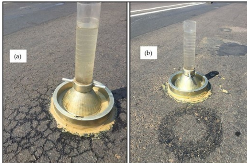
Figure 4: Marvil test on severely cracked road, (a) before application of a NPNS clear seal, showing water seeping out along the extensive network of cracks and, (b) after application of a clear seal
