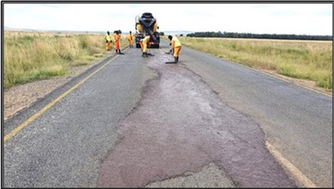
Figure 9: Filling of deformed areas on the road surface using a medium MC-NME slurry mix as a pre-treatment to address severe deformation before applying an anionic MC-NME slurry across the whole width of the lane and road
