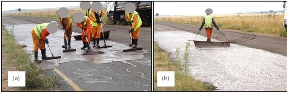
Figure 7: (a) Application of a labour-intensive anionic NME slurry seal to effectively provide a water-repellent new surfacing, preventing water ingress into the pavement structure on a severely cracked surfacing-restoring some riding quality; (b) A hessian drag-net is pulled over the slurry seal to provide even distribution and even texture to the slurry seal
