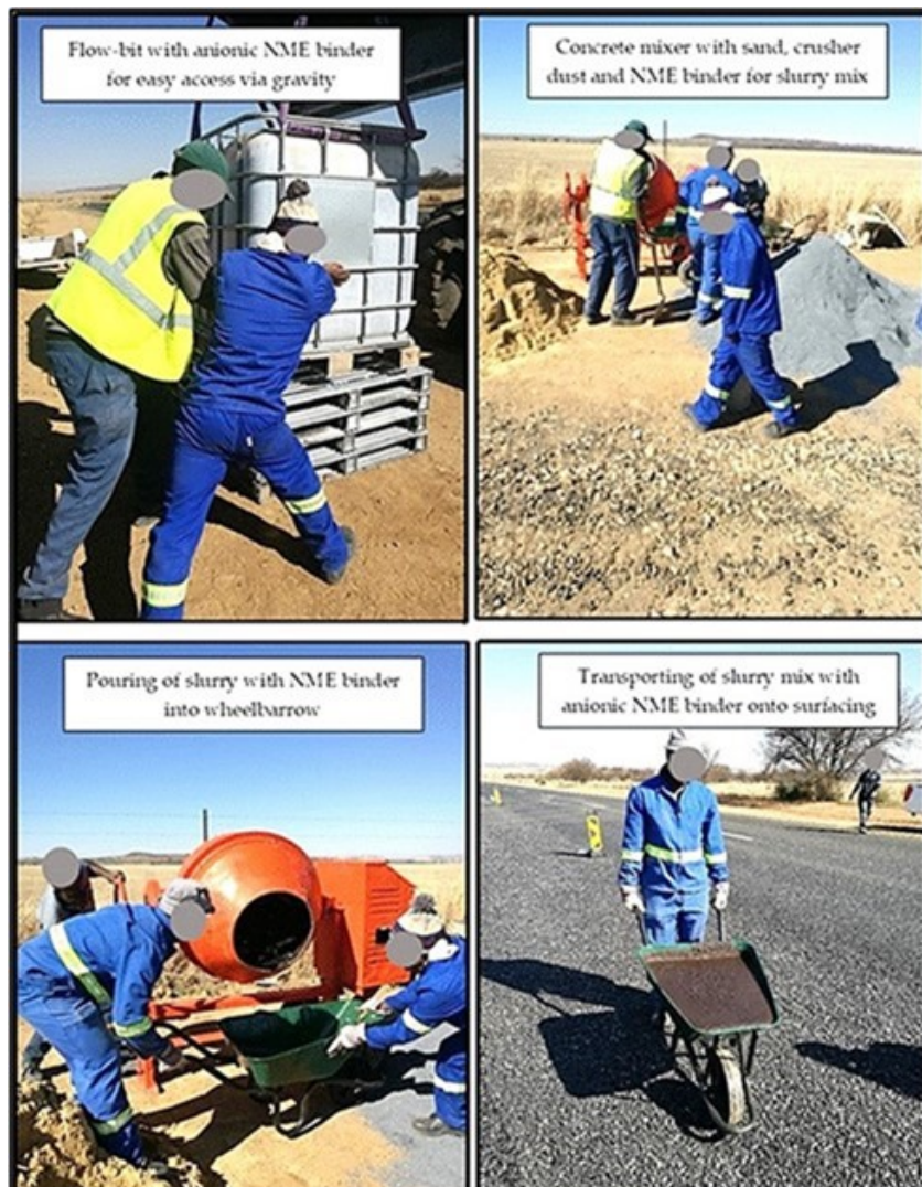
Figure 8: Labour-intensive roadside manufacturing of the slurry mix for an anionic NME binder slurry seal or a modified Cape seal using an anionic NME binder
