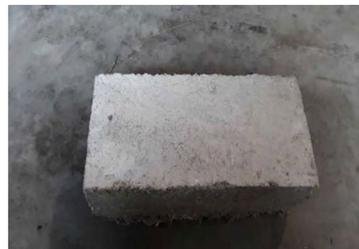
Moderate - When there is a greater deposit than under slight and covering up to 50% of the exposed area of the concrete surface but unaccompanied by powdering or flaking of the surface.
