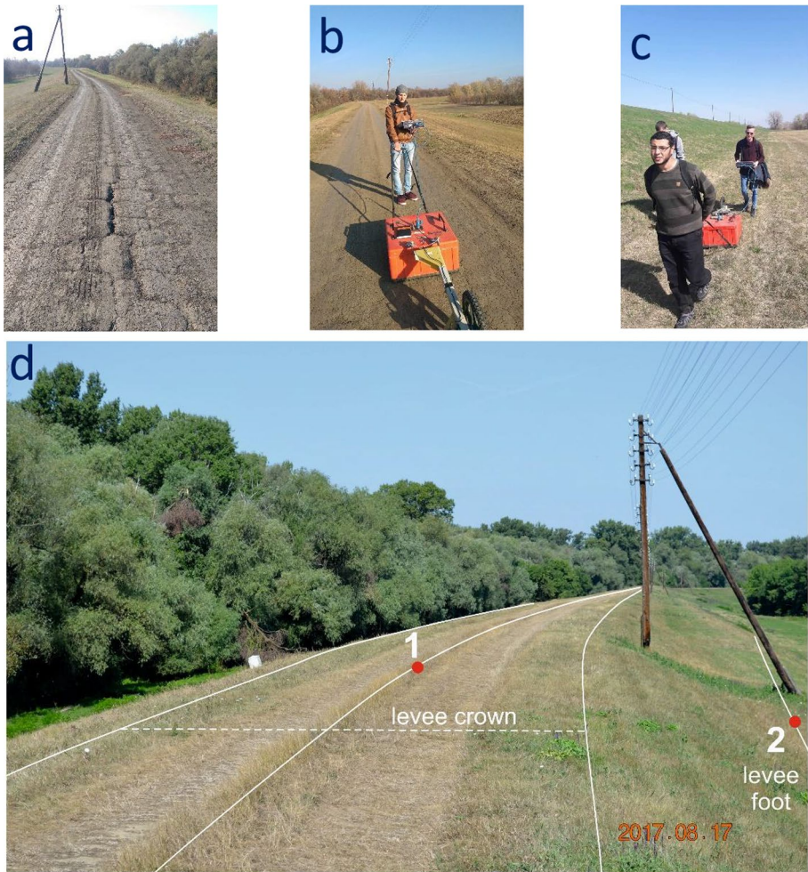
Fig. 3 a Tensile cracks on the levee crown, b GPR survey using SIR3000 attached to a 200-MHz shielded antenna on the levee crown, c GPR survey on the levee foot, and d location of GPS points measured on the levee crown and levee foot
