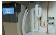
Typical under-sink water softener installation
