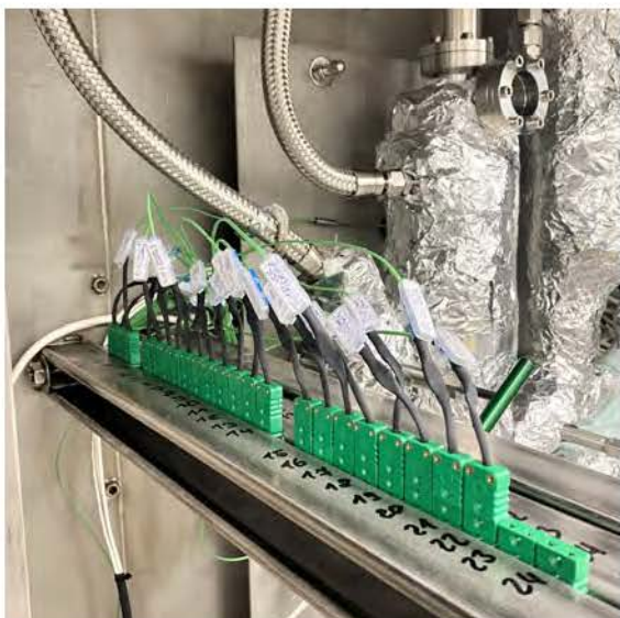
Fig. 8.10. Thermocouple connector strip mounted on the horizontal beam support in the center of the glove box.
