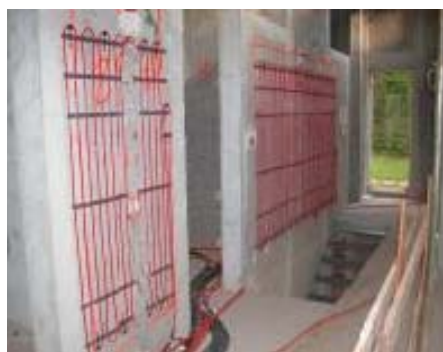
Figure 14. Wall heating system
