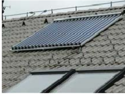
Figure 8. Fixed solar collectors
