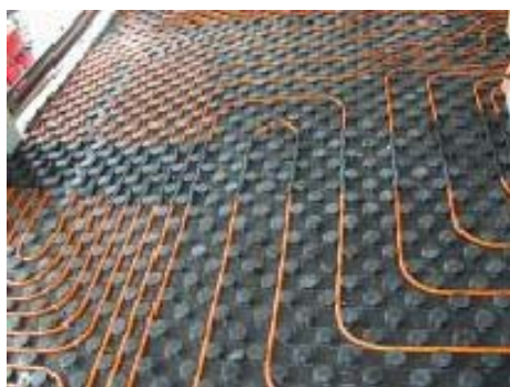
Figure 13. Underfloor heating system
