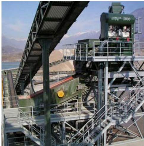
Figure 2. Technological circuit with installed ALLJIG ® jig by ALLMINERAL company [6]
