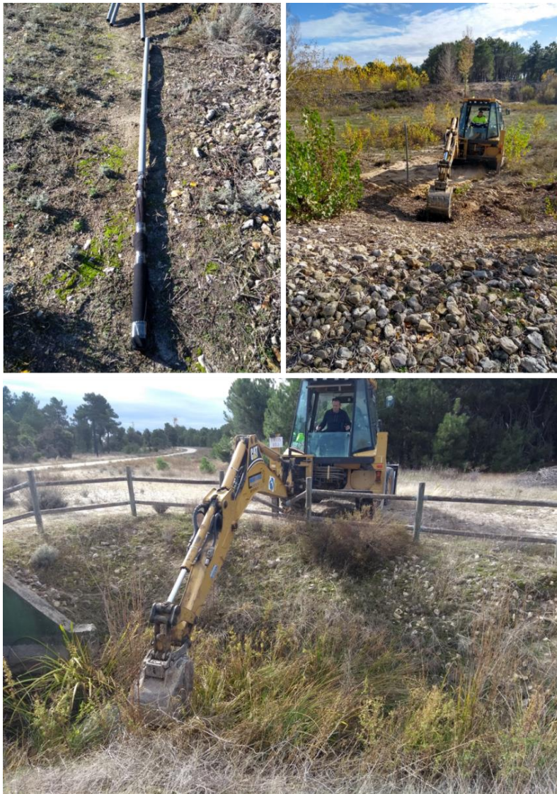
Figure 30. Fieldwork conducted in the study site to construct the monitoring piezometers and maintain infiltration infrastructure: a) slotted pipe with filtering fabric installed in one of the infiltration basins; b) Installation of the slotted pipe in La Laguna del Señor infiltration basin; and c) Maintenance of a small infiltration pond next to station the ZNS-3.
