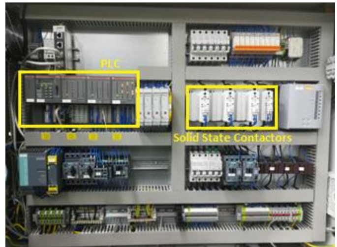
Figure 2. The appearance of the electrical control cabinet
