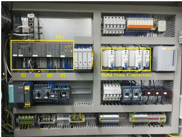
Fig. 6 The electrical control cabinet of conveyor belt furnace
