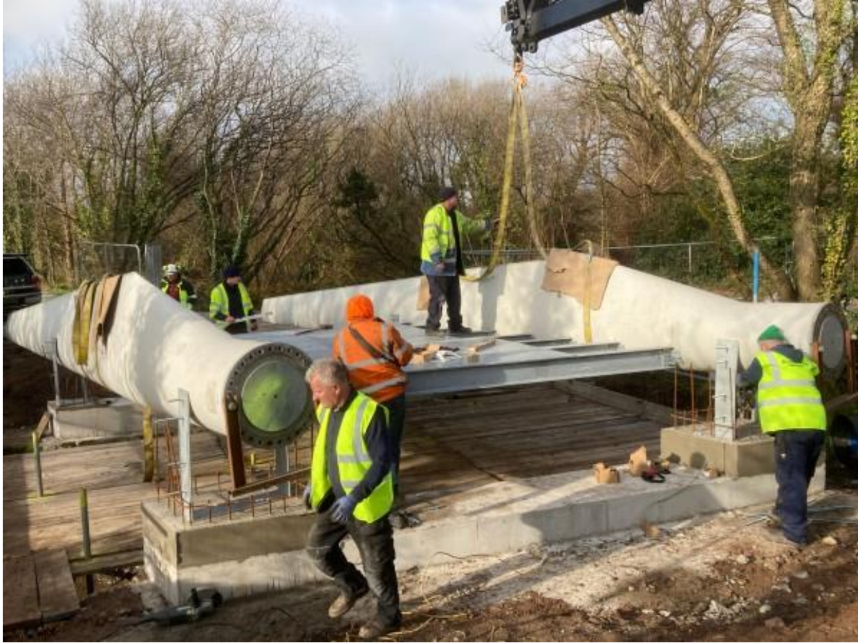
Figure 8. Wind turbine blades being used for the construction of a bridge in Ireland (Brandon, 2022).
